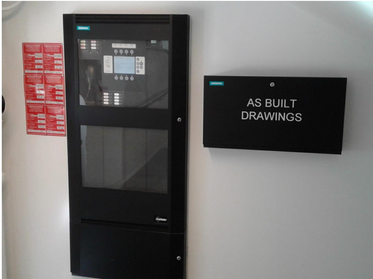
Figure 1. Fire Controller and Command Station at FHR 2014 South West Stair
