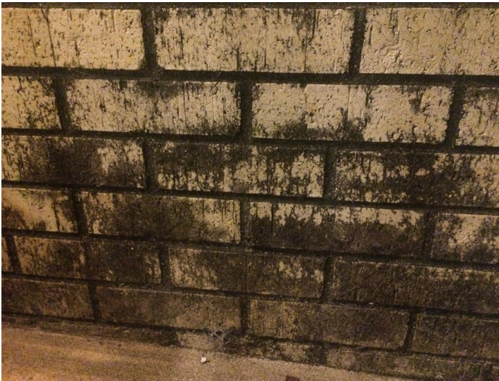
Figure 32. (below) sediment build-up from moisture run-off; field survey, November 30, 2017.
