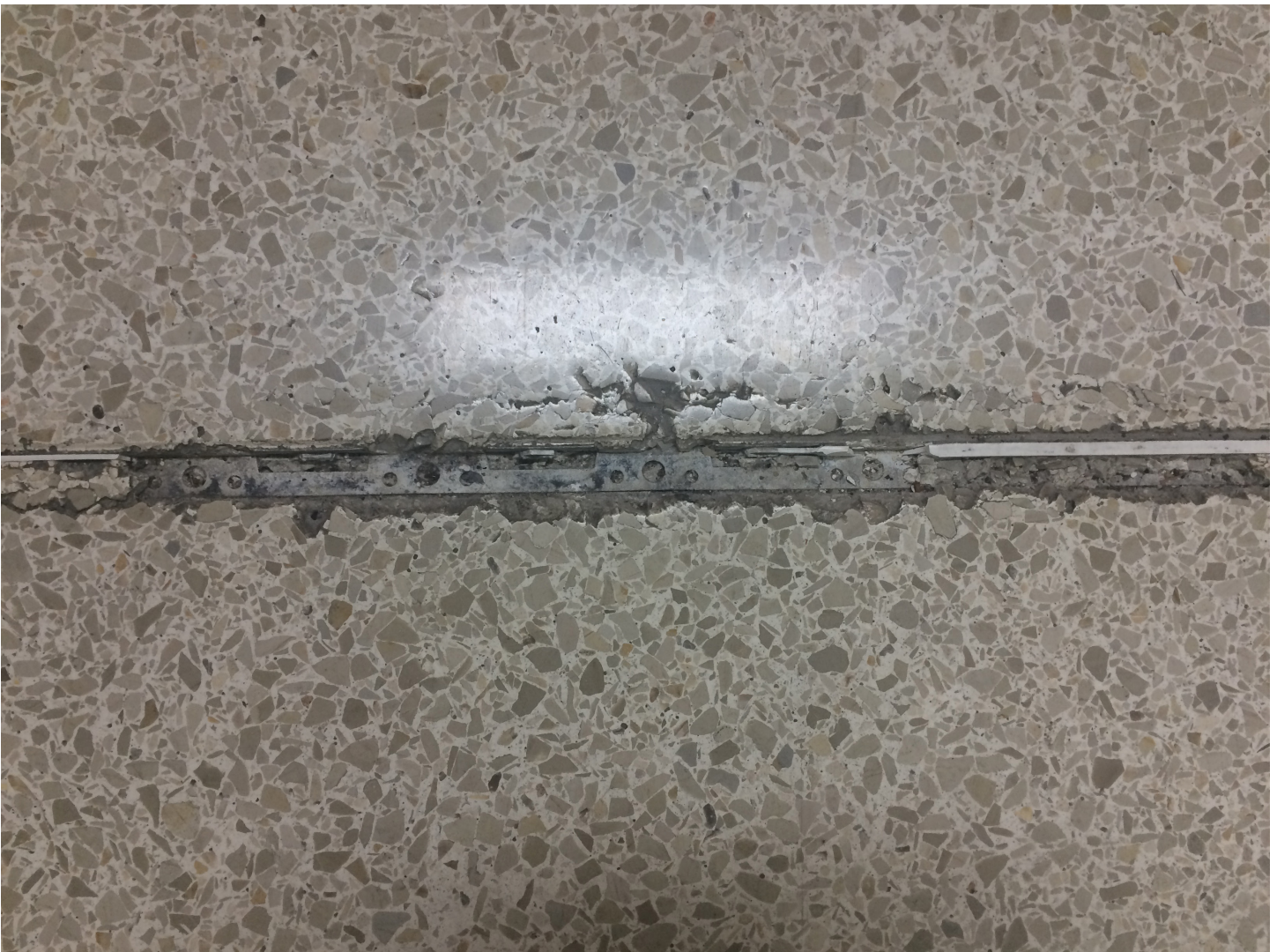
Figure 41. (below) damaged terrazzo, first floor; field survey, November 30, 2017.
