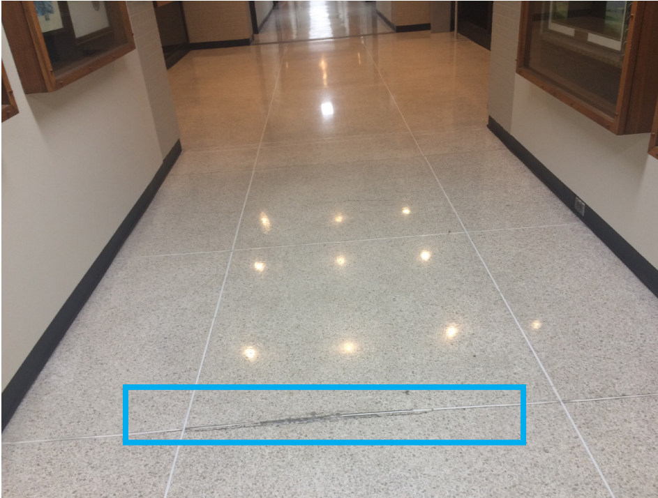
Figure 38. (top, page 30) damaged outlet, first floor; field survey, November 30, 2017.
