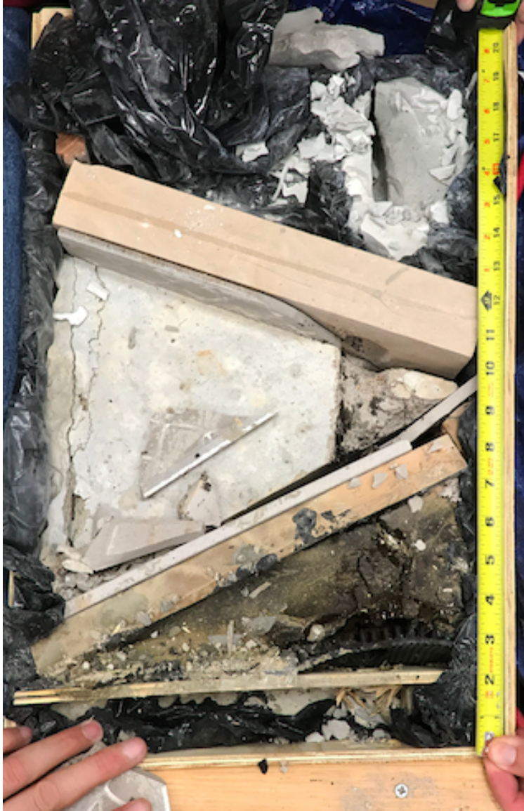
Figure 3.12: The rock sample after having been drilled. From top to bottom the formations encountered are soft cement (7 in) sandstone (2 in), granular cement (2.5 in), limestone tiles (1.5 in), asphalt (4in).
