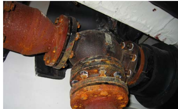
Fig.13 ice storage condition (2) electric valve
