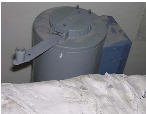
Fig.11 ice storage condition (1) electric valve
