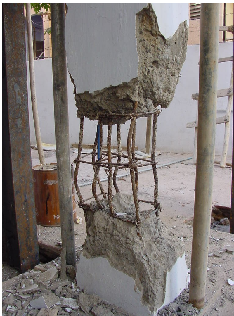
Figure 4 Column failure at 2001 Bhuj earthquake 3
